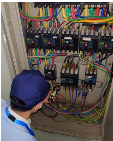
Power management project at Shanghai Suoguang Visual Products Co., Ltd.
