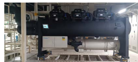
Chiller system installed at STT
