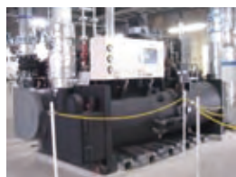
High-efficiency turbo chiller installed at Kisarazu TEC
