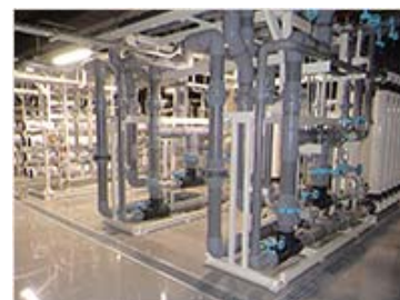
A wastewater recovery system for gas detoxification equipment
