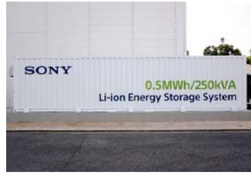
Large-scale storage battery system installed in Sony Energy Devices
