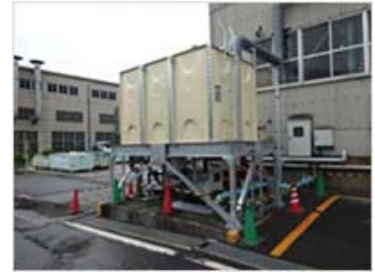
A rainwater storage tank next to the warehouse building
