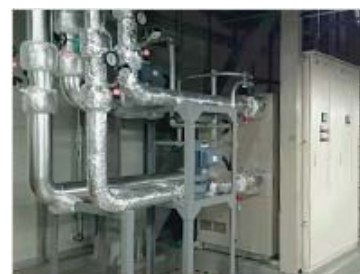
A highly efficient heat recovery system was installed in the pure water room
