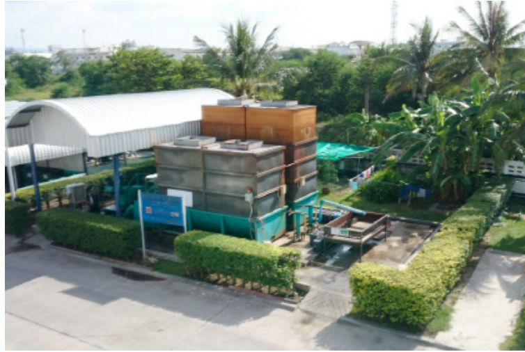
The biogas facility
