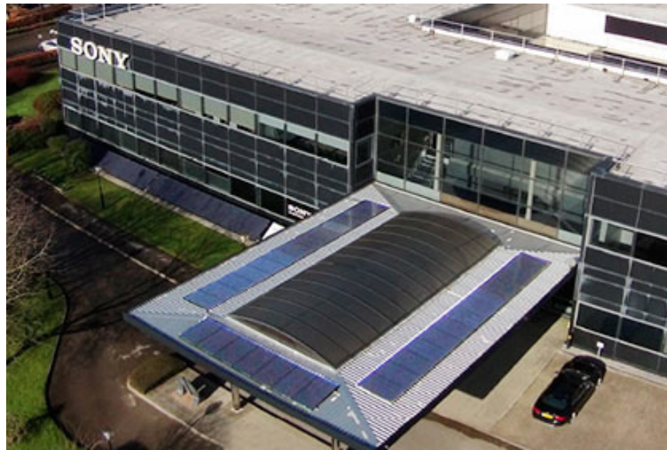
PV Solar Panels on the roof of the UK TEC
