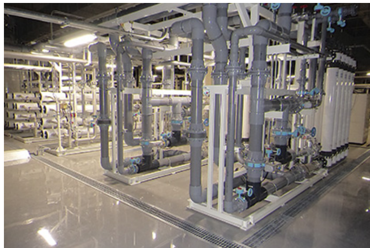
A wastewater recovery system for gas detoxification equipment
