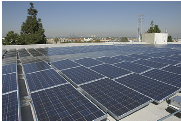
Solar power generation facility installed on the roof of SPE's headquarters
