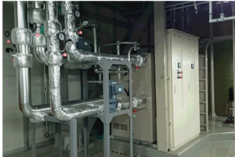
A highly efficient heat recovery system was installed in the pure water room
