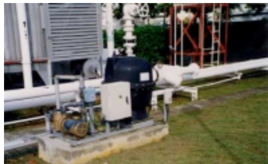
The cleaning water filter and circulation/recycling system for the cooling tower
