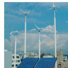
Rooftop wind and solar power generators
