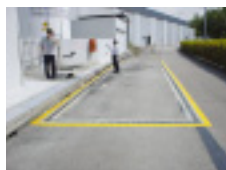
Wastewater pit installed in trailer yard to prevent leaks from fuel oil tanks Sony Display Device (Singapore)
